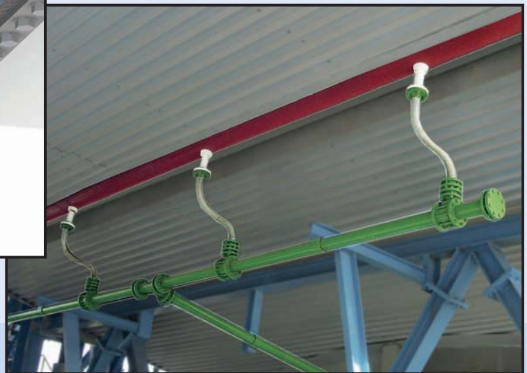
Fig. 3F: Manguera de inoxidable conectada a drenajes de PTFE Stainless steel hose connected to PTFE drain ports
